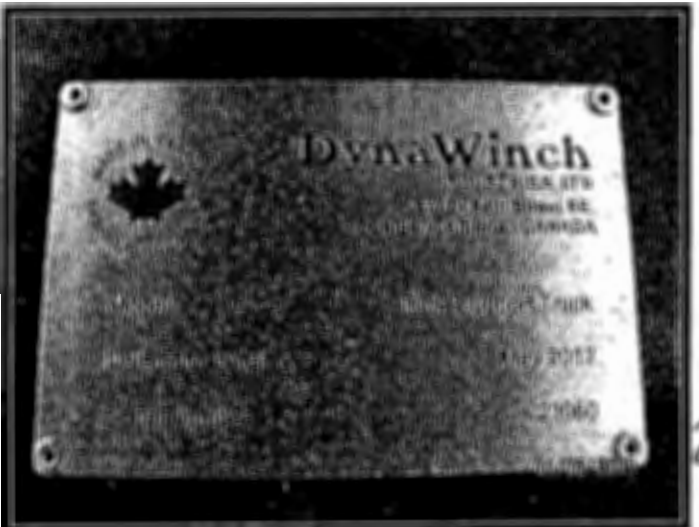
Accumulator ID Placard
