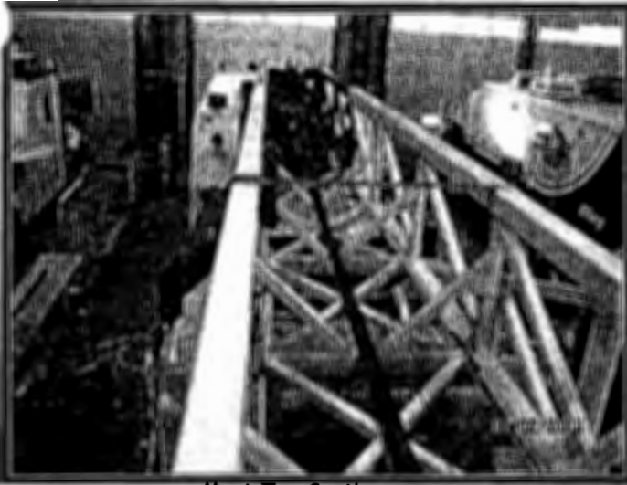
Mast Top Section
